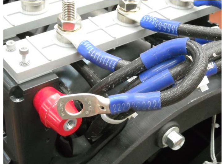
Fig.17 n.2 power cable on the isolator
